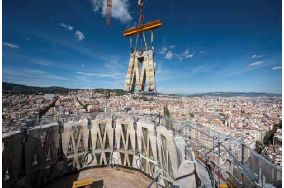
Fig. 7: Construction of central towers using prestressed stone panels reinforced by stainless steel columns joined with high-strength concrete (© Fundació Junta Constructora del Temple de la Sagrada Família)
