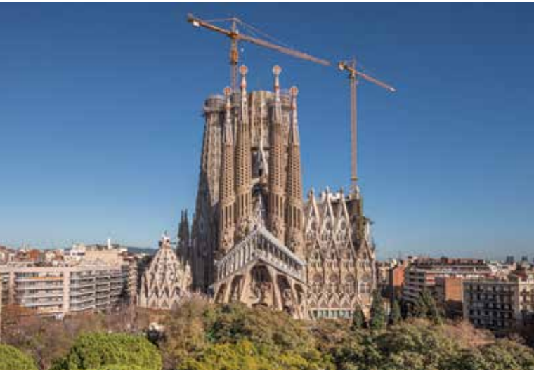
Fig. 2: The Passion façade features two 112 m (367 ft) bell towers flanked by two 102 m (334 ft) bell towers. Behind these, six more towers are under construction (© Fundació Junta Constructora del Temple de la Sagrada Família)
