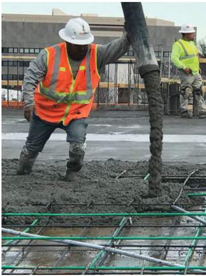
Well-designed mixes pump easily, are finishable, and meet all of the hardened specifications.
