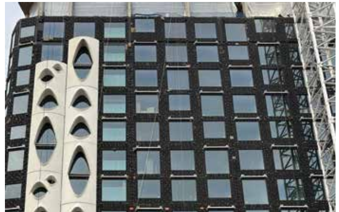
Fig. 6: The Populus hotel's façade during construction. The black areas are the weather wall's barrier membrane. The alternating metallic bands are high-strength galvanized steel "towel bars" for hanging the white GFRP panels (photo courtesy of Cannon Masonry)
